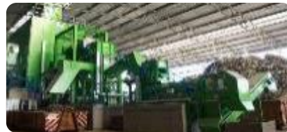
Gent: SRF production line and water treatment
