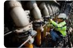
Biological water treatment
